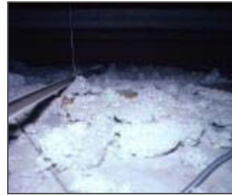
Debris from Fireproofing on Top of Ceiling
