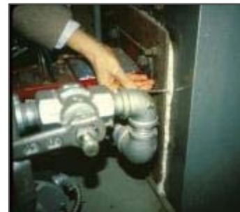
Roper Gasket at Boiler Plate
