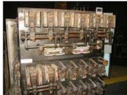
Transite Blocks in Elevator Switchgear
